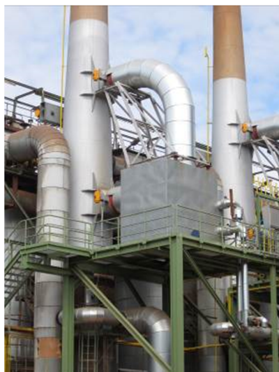
Figure 6. Heat recovery system at AOS.
